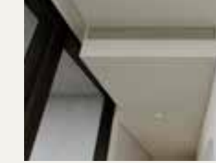
AIR CONDITIONING Outlet in bedrooms (available for 1, 2 and 3 bedroom units).
